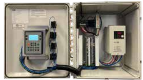
Inside Control Box
