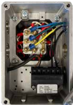
Internal view of sealed Motor/Brake Junction Box
